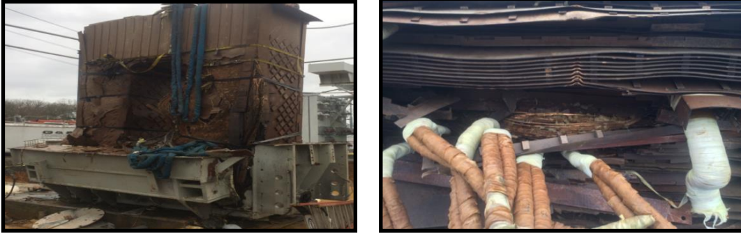
Figure 1. Transformer failure in a recent event
