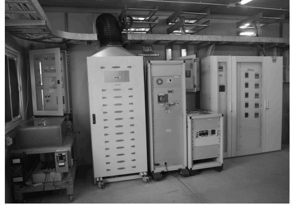
Fig. 3. Photo of the RSE's DC microgrid.
