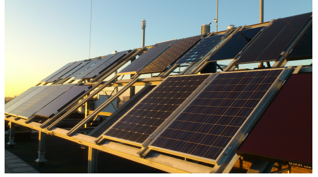
Fig. 1: Photograph of the Utrecht Photovoltaic Outdoor Test facility (UPOT). Photo courtesy of Arjen de Waal. (Best viewed in color)
