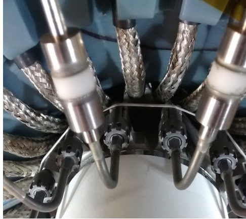
Figure 67: The cooling line electrical break in the ID end flange service region.
