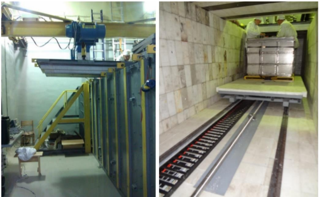
FIG.3. General view of passive shielding: from the outside and inside. The range of detector dislocation is 6 - 12 m from the reactor core center.
