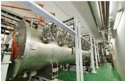
FIG. 21: The two cryomodules of Injector-I installed in the tunnel
