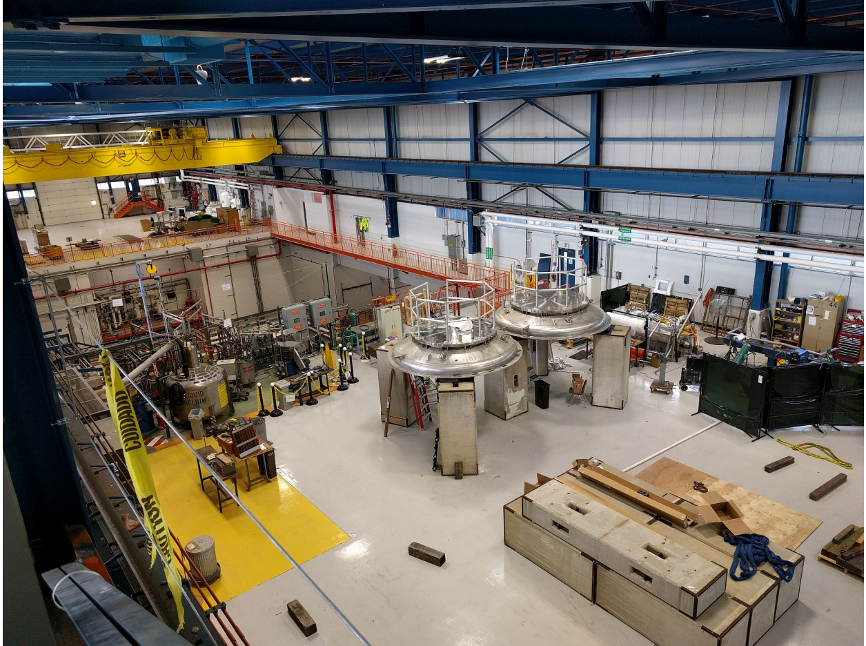
Figure 2 - Interior of the HAB. The cryogenic plant can be seen in the center left. Approximately 6,000 ft 2 on either side of the center pit
