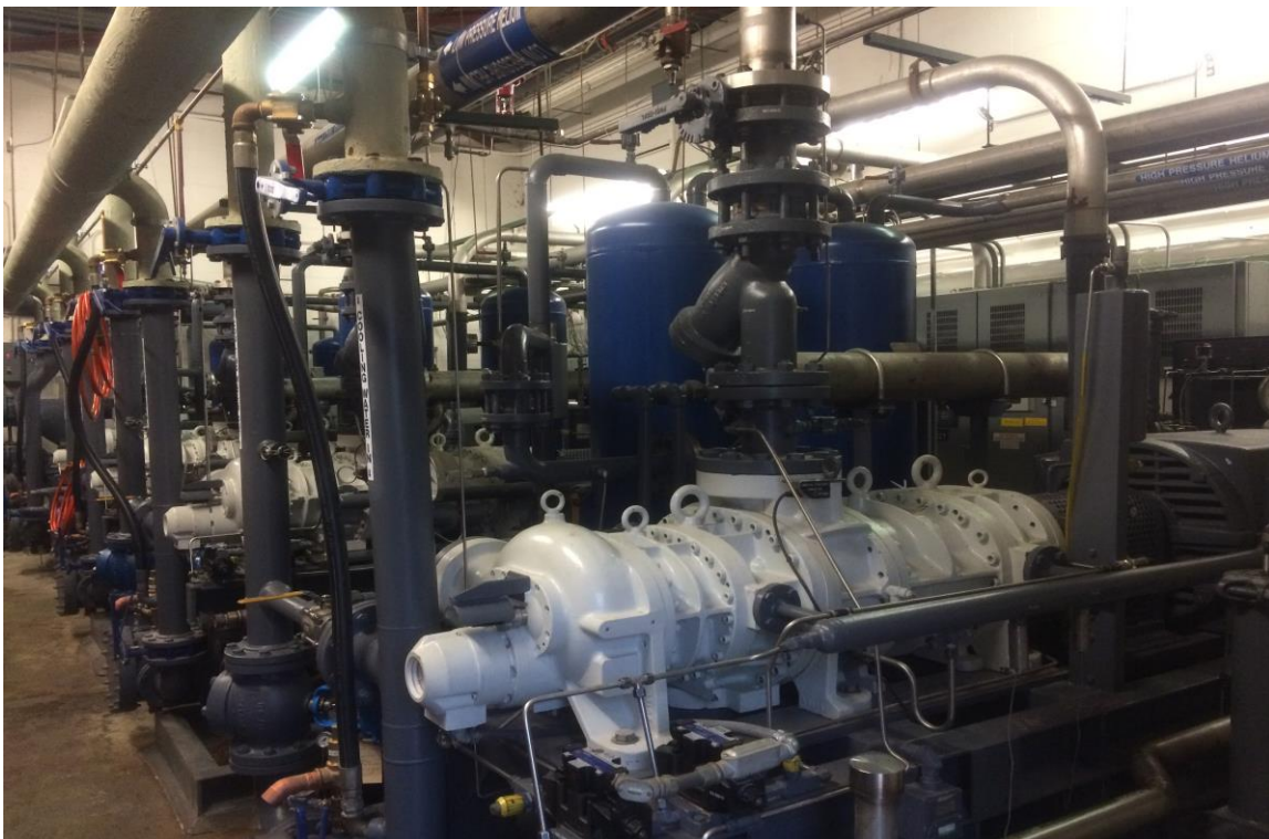
FIGURE 2. A0 Warm Compressor Room
