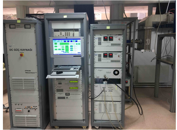
Figure 7: SPP PSU in use. The left rack has the DC power supply, the central rack has the controller and the master signal generator, and the right rack has the power supplies for the tetrode gates, the first amplification stage and the output to the Tetrode amplifier rack.
