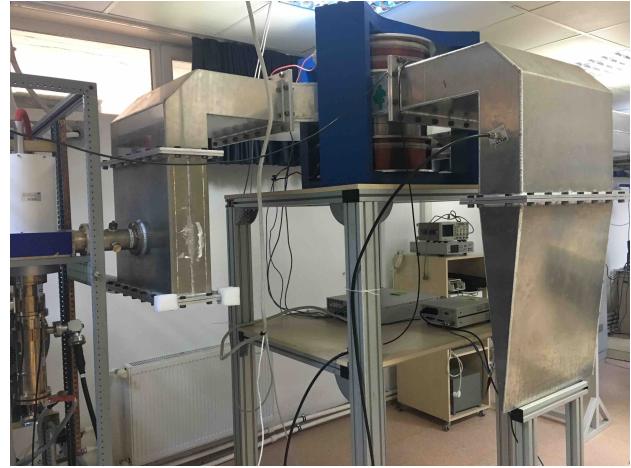
Figure 20: 352.21 MHz waveguide circulator as it is installed in the RF transmission line. Note that the connection to the RF PSU (port-1 one left side) was made with a 3 1/8" rigid coaxial line. The electromagnet, PSU and the gauss-meter are right below the circulator.
