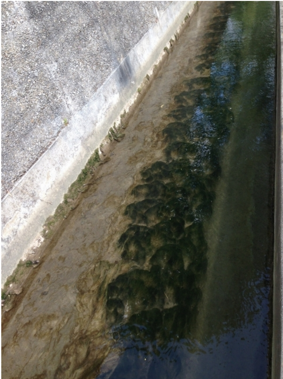
Figure 4: Concrete channel with some sediment transport and presence of longitudinal vegetation patterns; Picture credits: Paolo Perona
