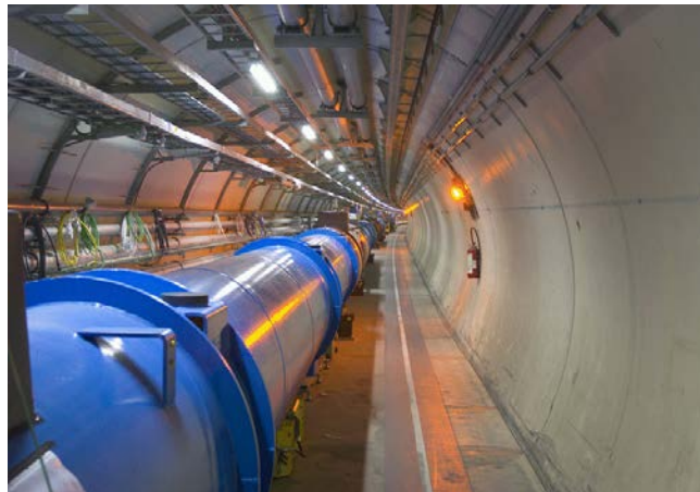
Fig. 5: The LHC tunnel with the dipole cryostats. The normalized bending force, represented by the radius of \rho = 2.5 km, is hardly visible.
