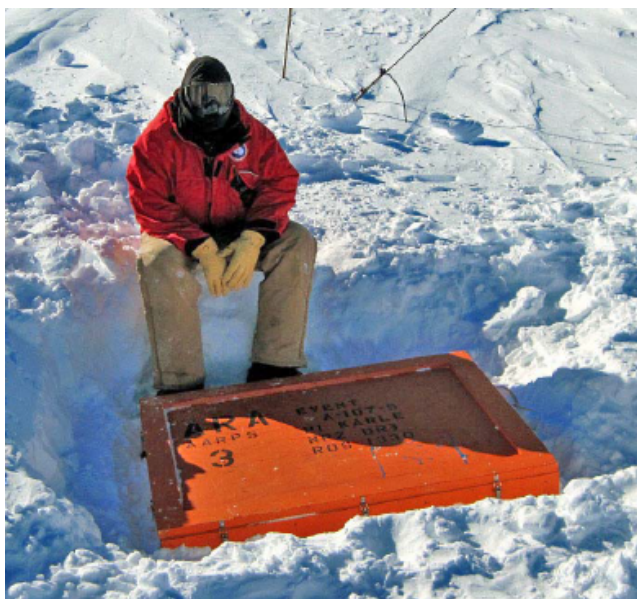
Figure 10: Instrument box installed. The boxes were buried just below the ice surface, helping to shield the system from extreme temperatures. This resulted in added difficulty when performing maintenance or troubleshooting by requiring ice and snow removal for access.
