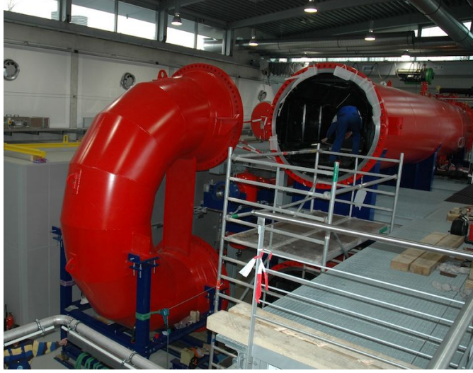
FIG. 5. One of two elbows is removed and reveals the cross section of the tunnel.
