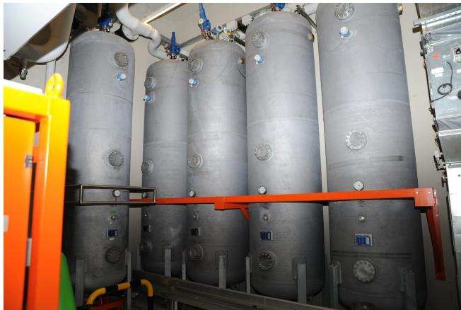
FIG. 9. Storage tanks, in which the SF 6 is stored in liquid form.
