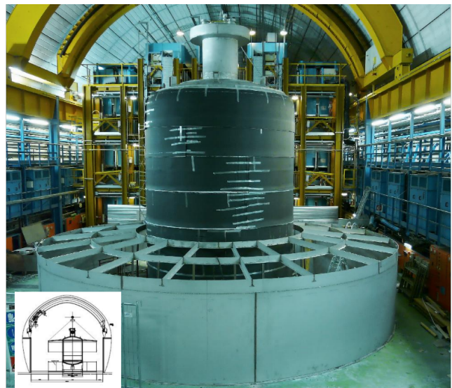
Fig. 7 The water tank under construction in Hall A of LNGS in front of the LVD detector. The inset shows how the tank is assembled from top to bottom. The hall crane lifts the upper part to which another cylinder segment of about 2 m height is welded. The cryostat in the center is protected by a black foamed plastic during the construction of the water tank.
