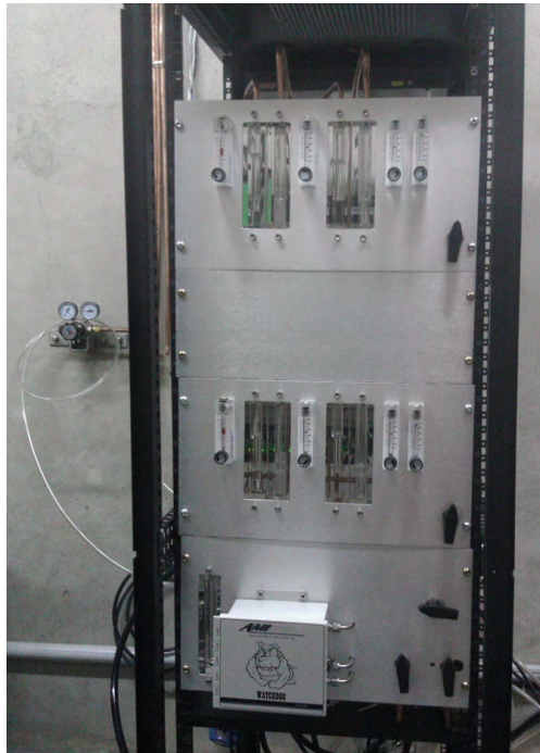
Figure 13. A gas rack for two ADs.
