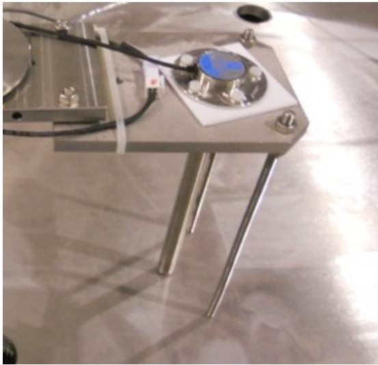
(a) A stainless steel capacitive liquid level sensor, located in a mineral oil overflow tank.
