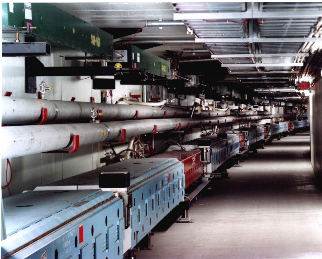
Figure 8: The completed Main Injector (bottom) and Recycler (top) within their shared enclosure. Note the absence of any electrical or water connections to the Recycler magnets!
