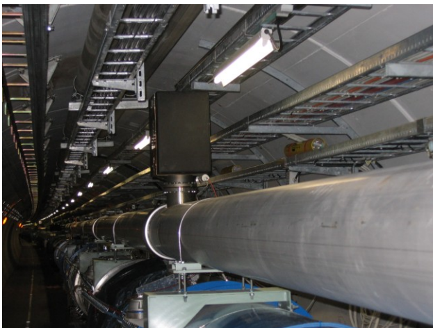
Figure 3. LHC dump line above the LHC
