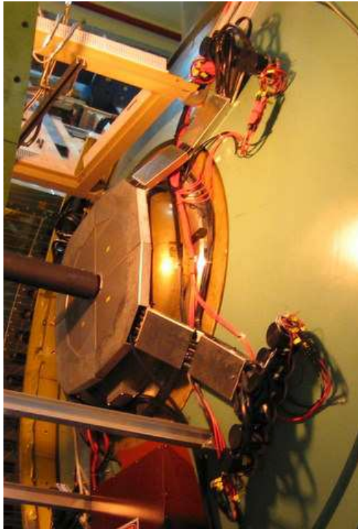
Figure 10: Picture of the RXNP's north half installed on the Cu nosecone of PHENIX's central magnet prior to the installation of the HBD.
