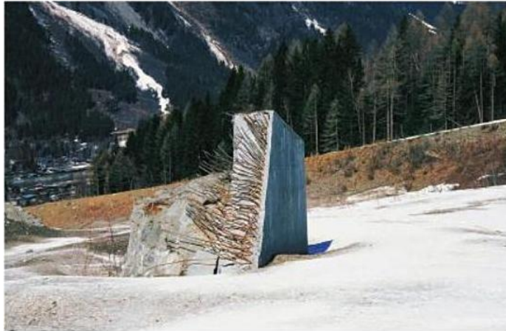
FIGURE 2. Protecting wall in armed concrete at Tacconnaz (Haute-Savoie, France) destroyed by the powder-snow avalanche of the 11 February 1999. The height is 7 m and the thickness is 1.5 m (Photo by C. Ancey).
