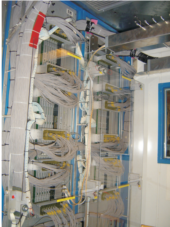
Figure 1: Details of the installed hardware in the electronic trailer of the H1 experiment: View of the Jet Trigger ADC-Calculation-Storage unit composed of 8 crates, one for each of the 8 octants of the LAr calorimeter. The system receives the analog trigger towers and transfers the digitized signals to the Bump Finder Unit via a bit-serial link.
