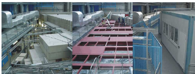
FIG. 4: Photographs taken from the same position in the ESR Experimental Hall and showing the construction of the HITRAP platform. Left: situation in 2004 before construction. Middle: situation in 2005 when the platform was erected for the huts housing the electronics of the HITRAP facility and of the the HITRAP experiments, for RF power supplies and other devices. Right panel: situation in 2006 when the platform is ready, the huts are in place, and the installations are almost completed.
